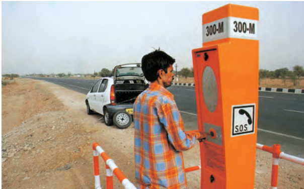
Fig. 7.10 : Emergency call box on NH-48
